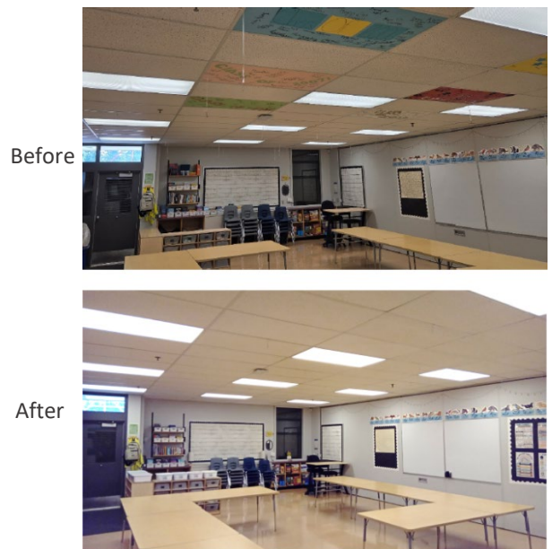
Figure 8: Lighting and Controls Upgrade at Glenwood Elementary
