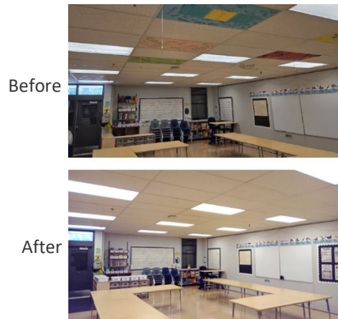
Figure 5: Lighting and Controls Upgrade at Glenwood Elementary
